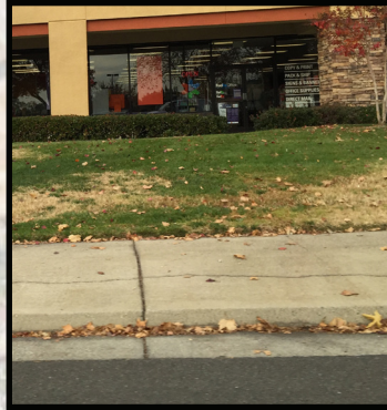
Heavy evidence of runoff
